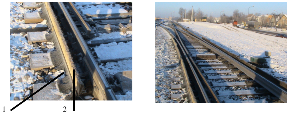
Fig. 2. The protection system of brushes from snow installed in the switch of Šiauliai railway station: 1 – lower part of brushes; 2 – upper part of brushes
