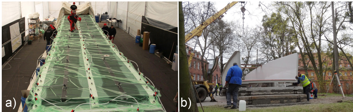
Fig. 11. a. Production of the footbridge; b. Structure assembly at Gdańsk University of Technology campus
