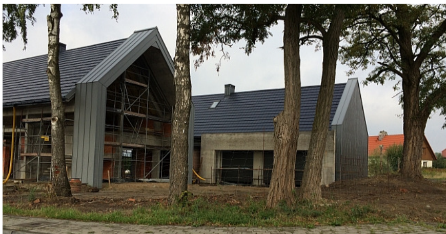
Fig 10. Modern residential development in Warmia and Mazury – construction stage (Source: Authors' own elaboration)
