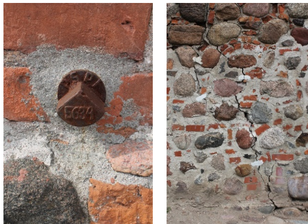
Fig. 8. Mark Num. 5634 on the left; on the right – visible crack on Grand Duke Palace
