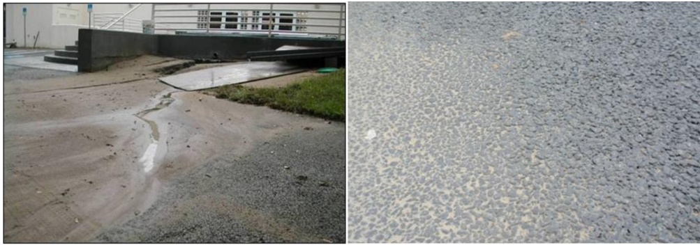
Fig. 4. Clogging caused by surrounding unplanted area, common clogging failure caused by surface runoff (Tong 2011)
